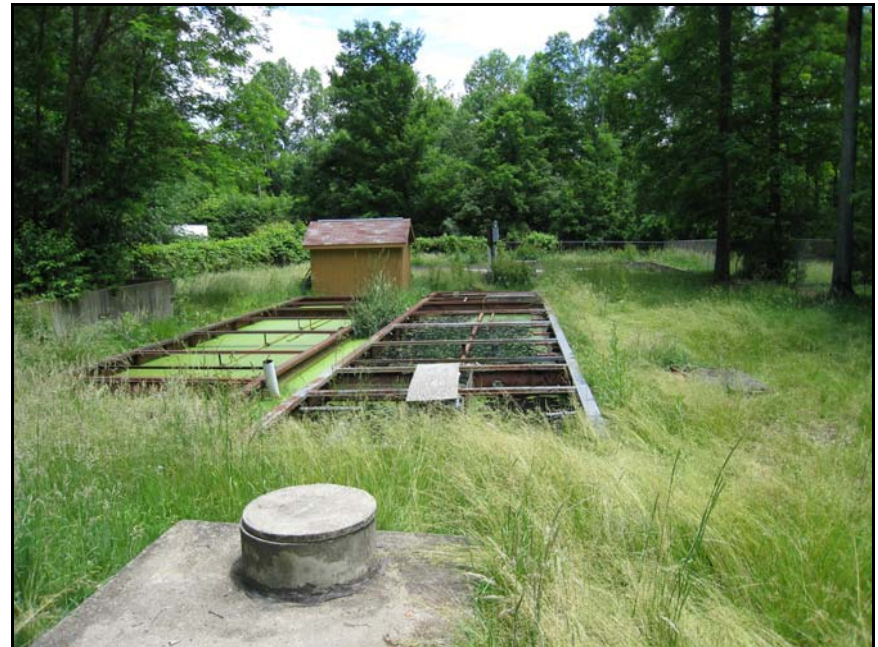
SEWAGE TREATMENT PLANT Winterized & Current EPA Certified
